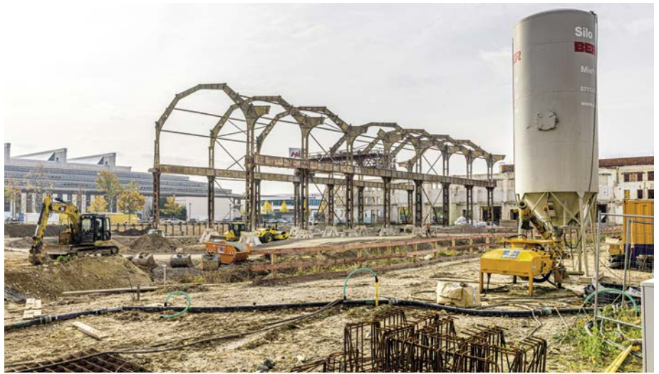
From old trade fair to new economy: A ~14,000 m 2 large complex with upscale lab, office and co-working spaces is being built for 62 million euros on the historic foundations of Trade Fair Hall 12 (a former machine tool hall on the BioCity Campus). It will serve as a new innovation center for smart health and life science companies.
